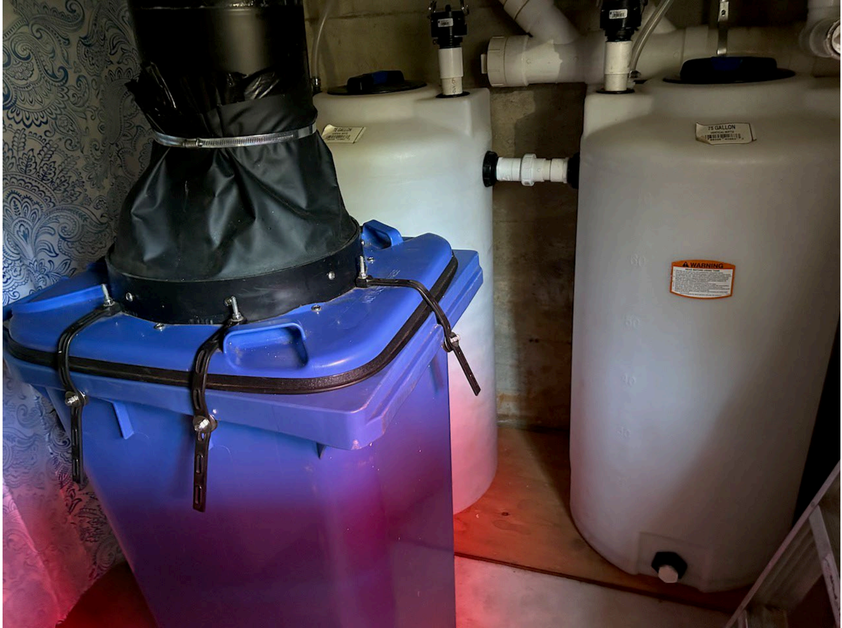
active bin #2 urine storage tanks
