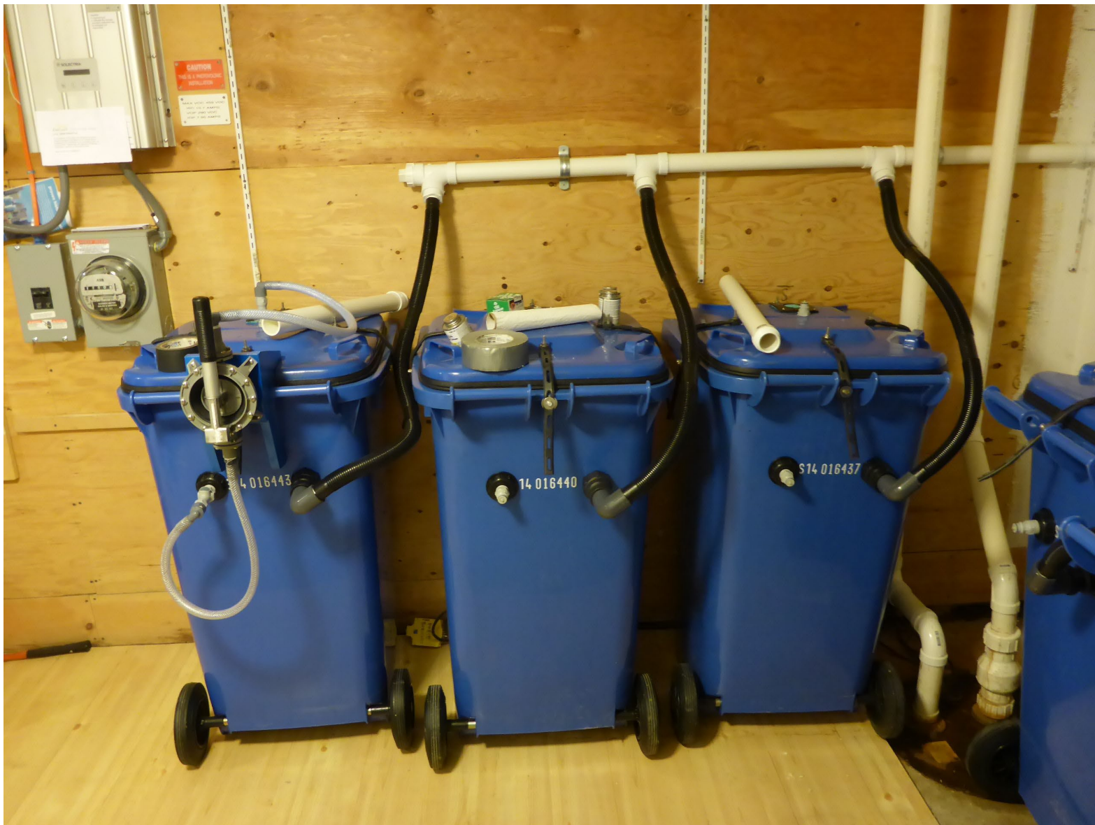
“resting bins” inside, with airlines to fan and chimney
